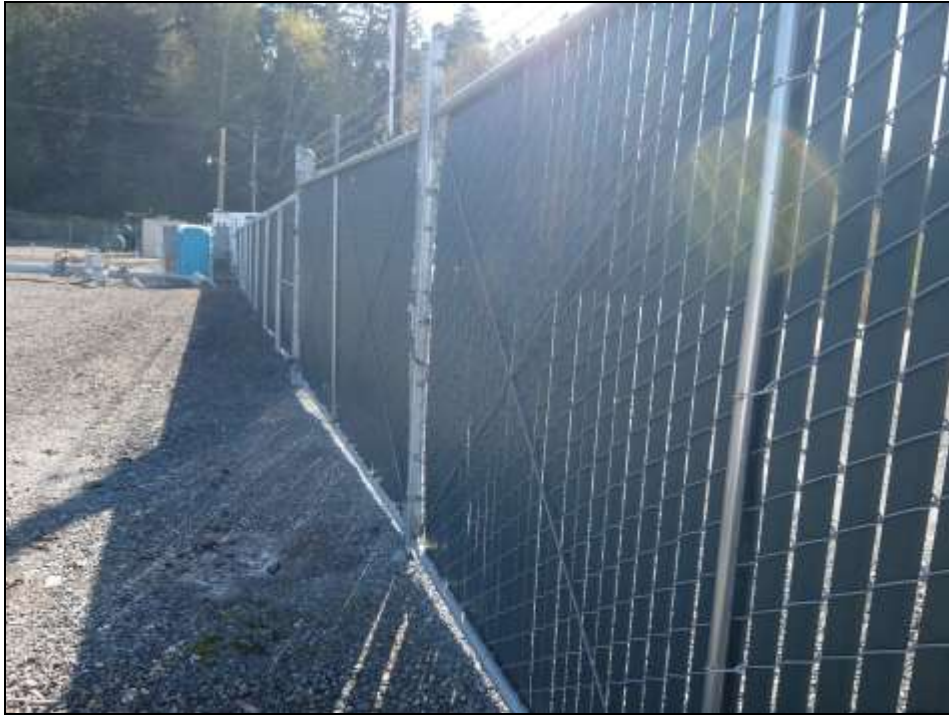
PHOTO THREE: EASTERLY VIEW OF IMPACTED FENCE
