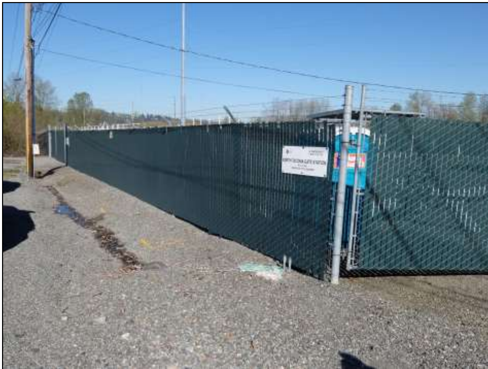
PHOTO SIX: WESTERLY VIEW OF IMPACTED FENCE/GATE
