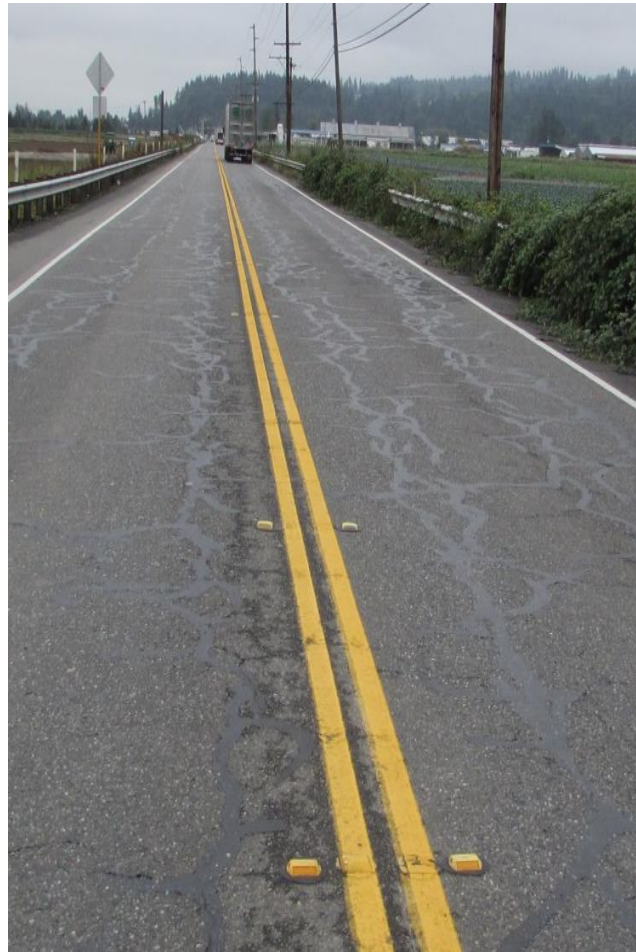
Poor Condition Road
