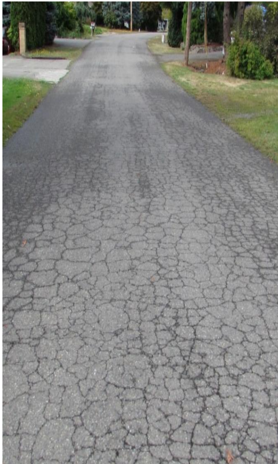
Very Poor Condition Road
