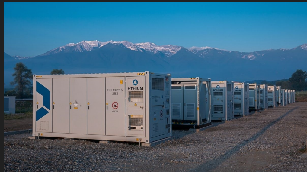
55 Mwh BESS goes live in Bulgaria https://www.pv-magazine.com
