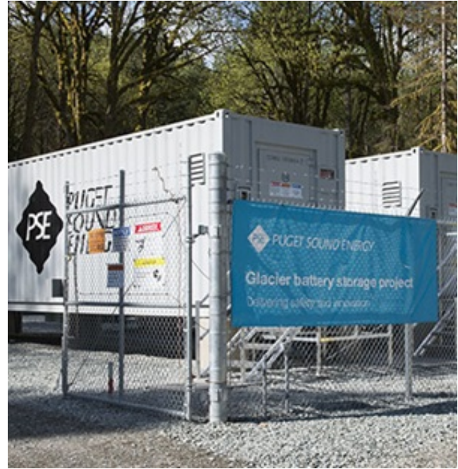
The Glacier battery storage project.
