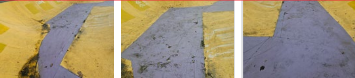
Damaged flat bottom, dangerous surface. Remove and replace.
