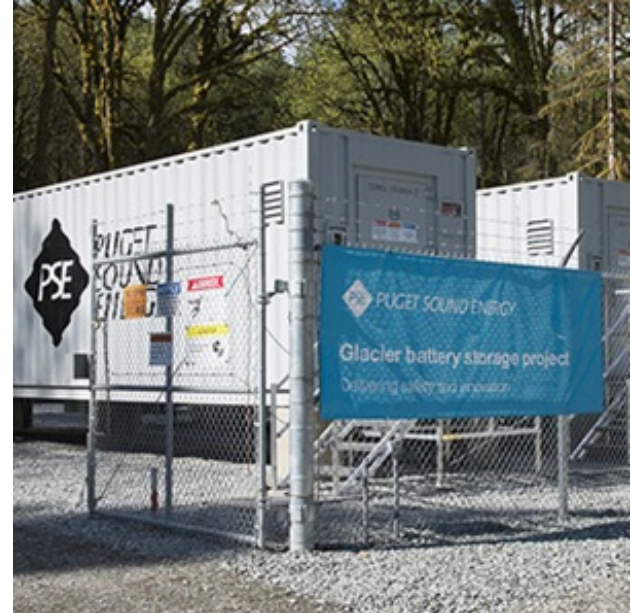
The Glacier battery storage project, a 2 MW/4.4 MWh lithium-ion system.
