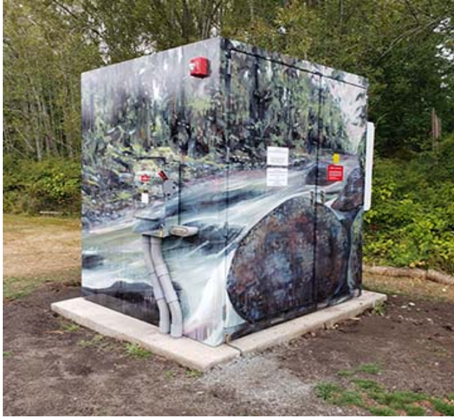
PSE installed a solar array and battery at the Samish Island Fire Station in 2023.
