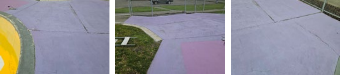
Dangerous seams and cracks. Unrepairable. Remove and replace.
