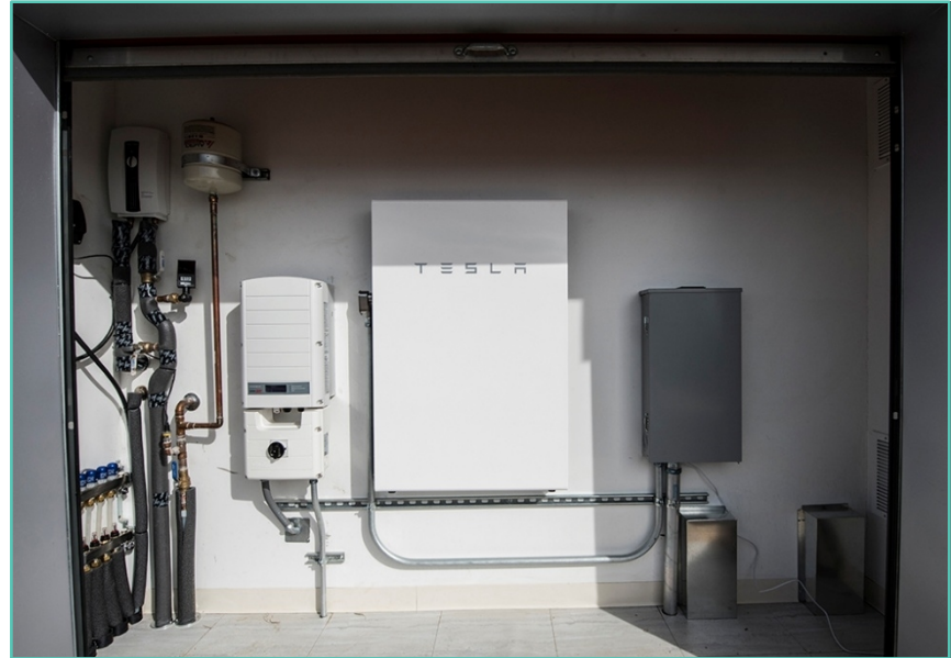
Example indoor Tesla battery wall charger
