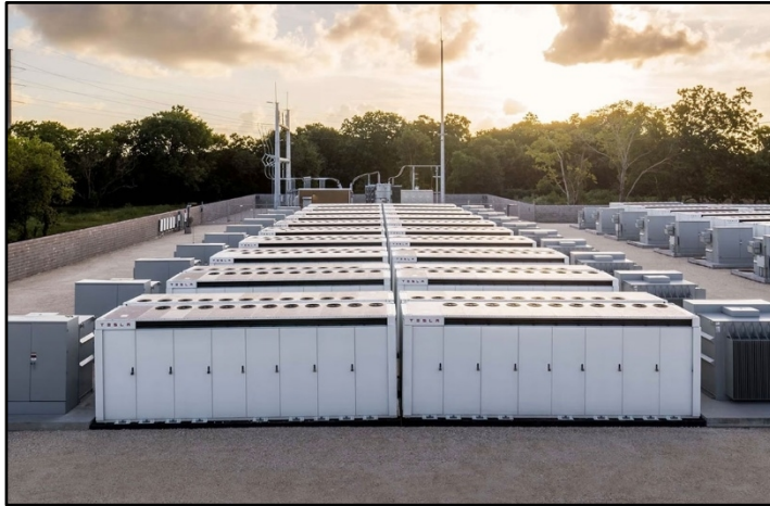
Example Utility grid-scale BESS facility
