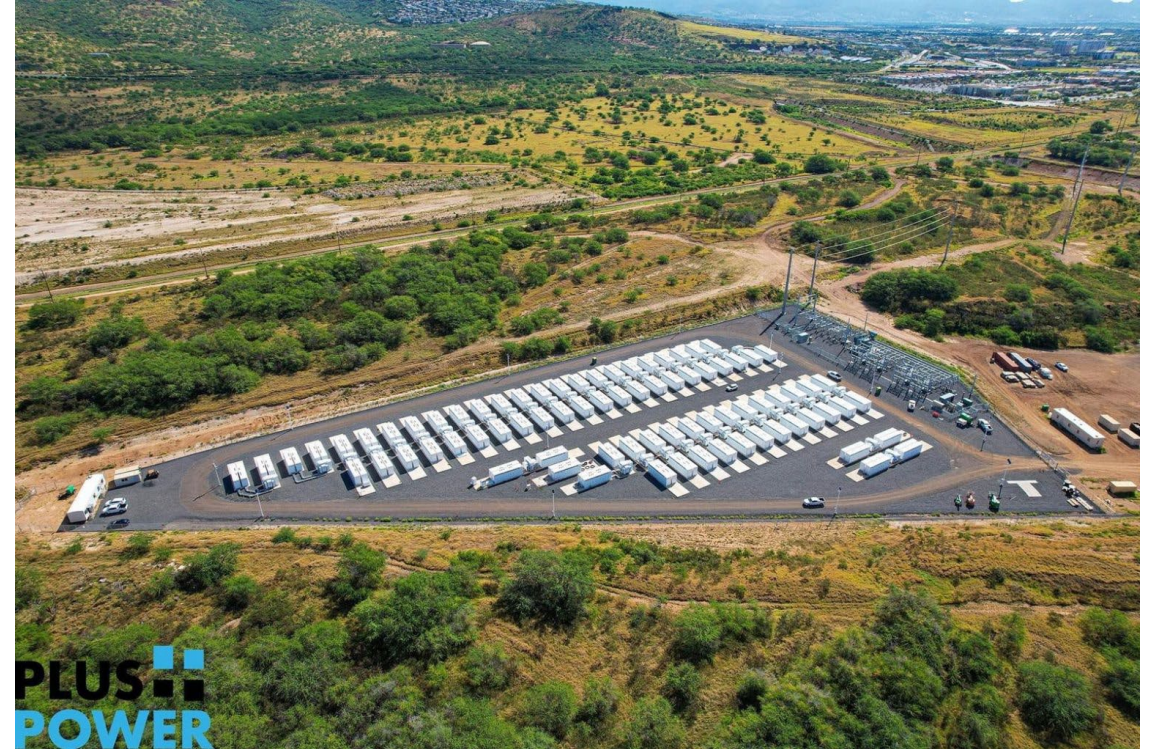
BESS site facility. Credit: Plus Power
