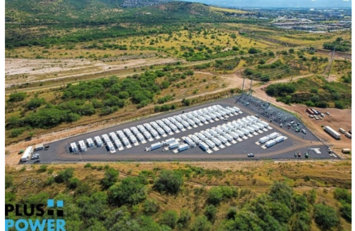
BESS site facility. Credit: Plus Power
