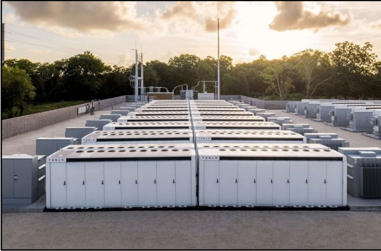
Utility grid-scale BESS facility
