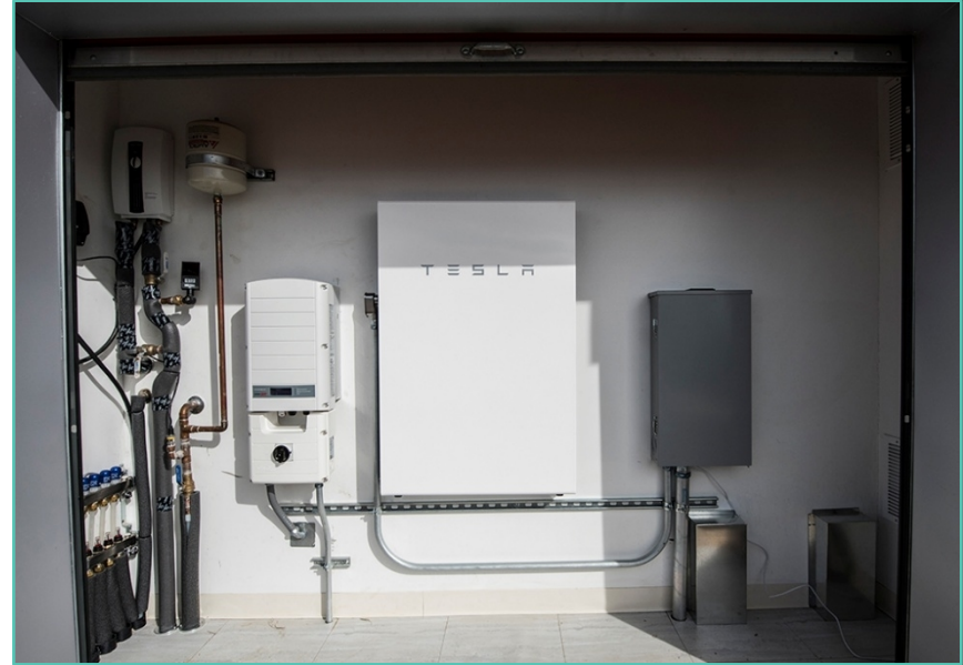
Example indoor Tesla battery wall charger
