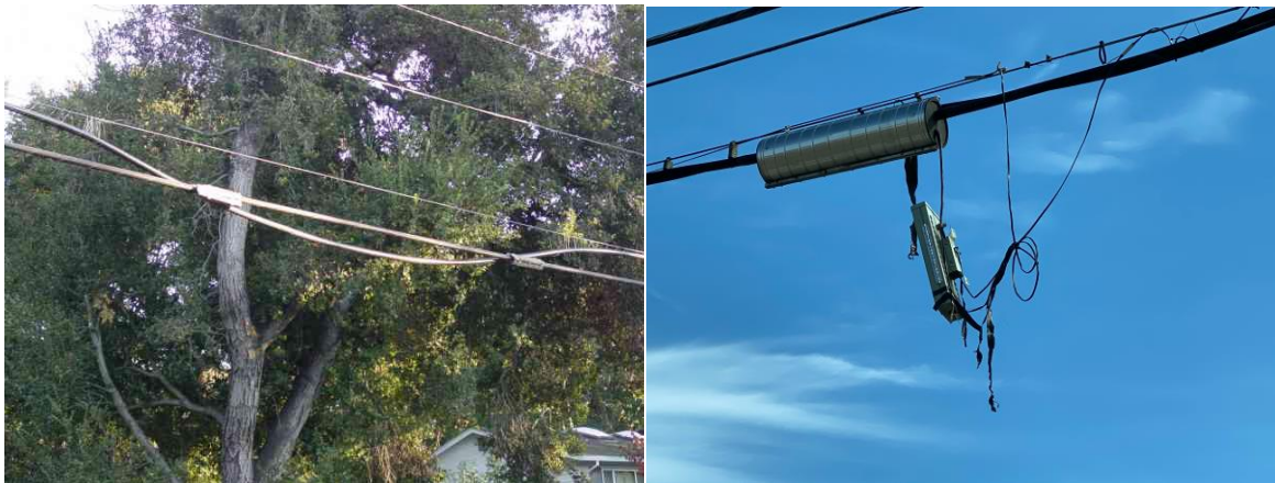
Figure 16 - Failed Aerial Lashing
