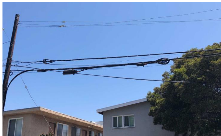
Figure 12- Aerial Cable with Splice Case and Snowshoe
